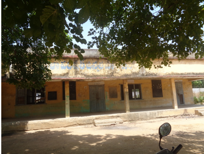
ZPHS School Building in dilapidated state at Madhavaram Village
