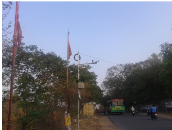
CCTV Camera at BDL Gate
