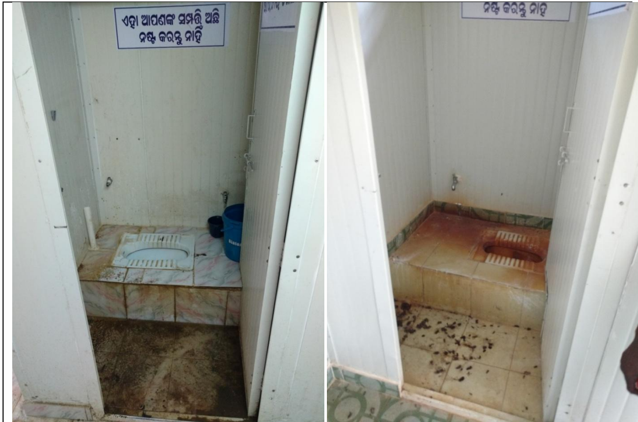
Figure 14 : Condition of the BDL supported Bio-Toilets
