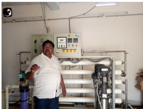
R.O Water Plant Machinery
