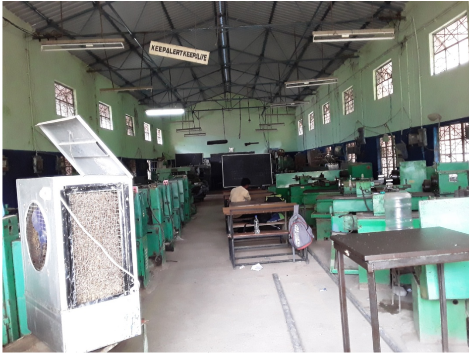
Renovation of workshop by removing of Asbestos sheet and laying new Galvanized Sheet
