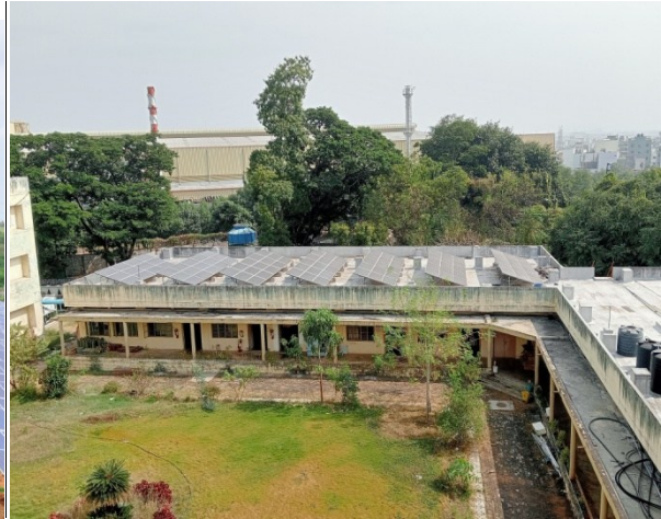
Rooftop Solar Power Plant
