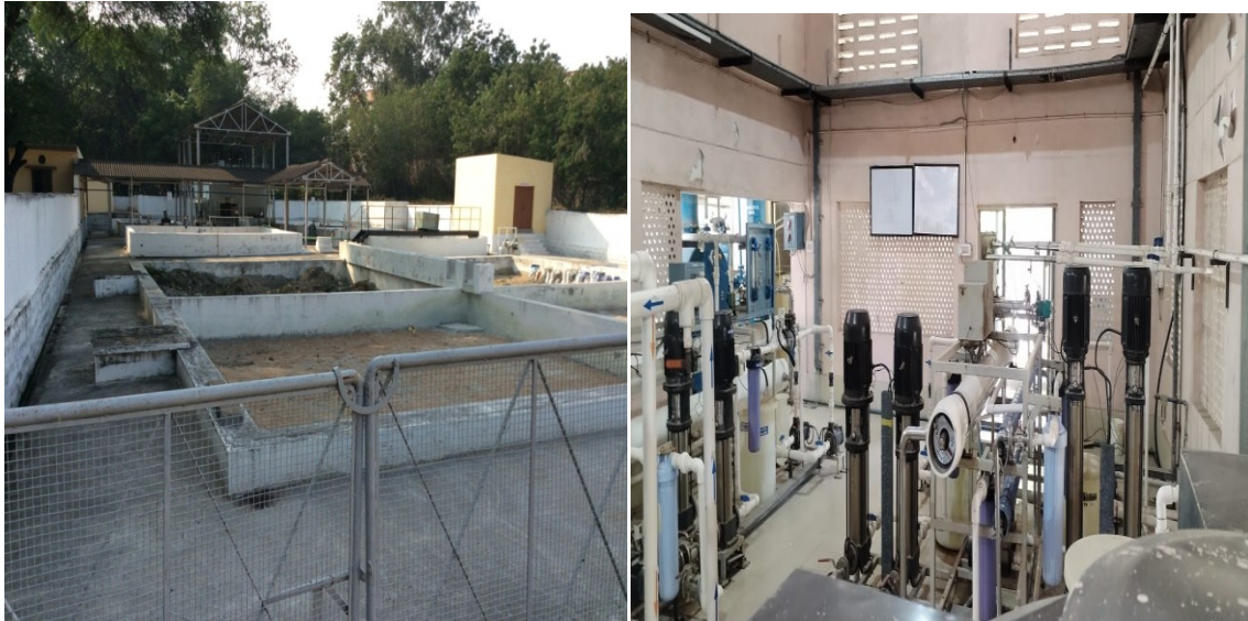
Effluent Treatment Plants
