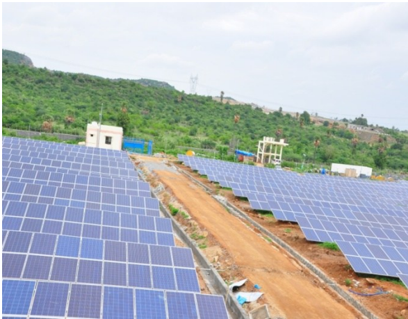
Land Based Solar Power Plant
