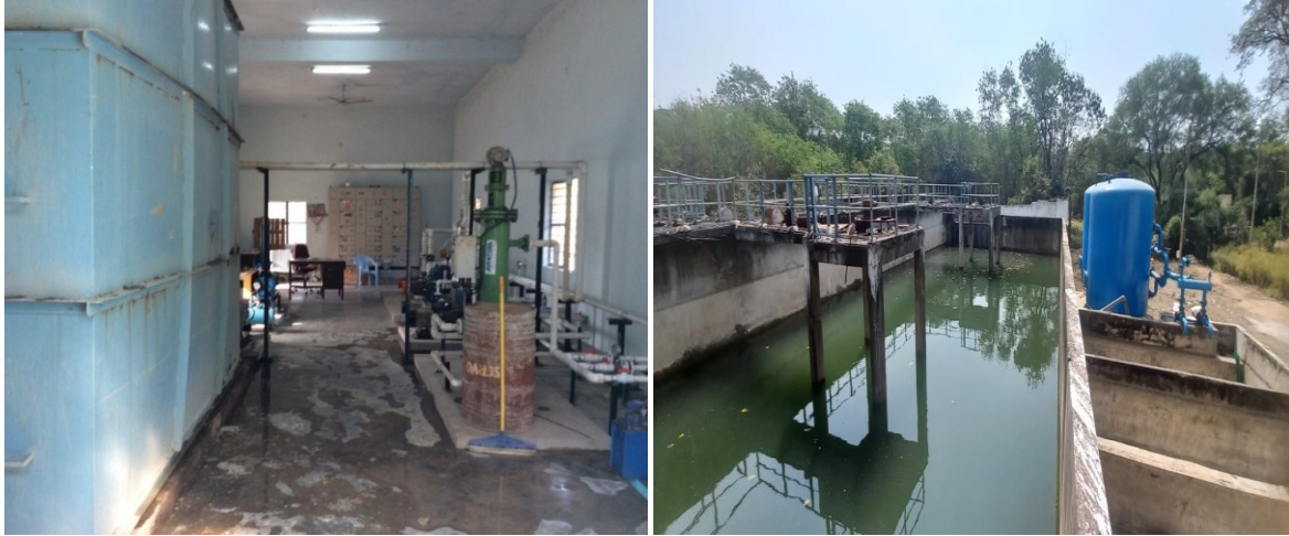
Sewage Treatment Plants
