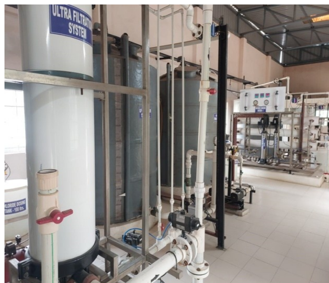
RO Plant at ETP Outlet
